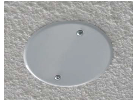
Ceiling Electrical Box
