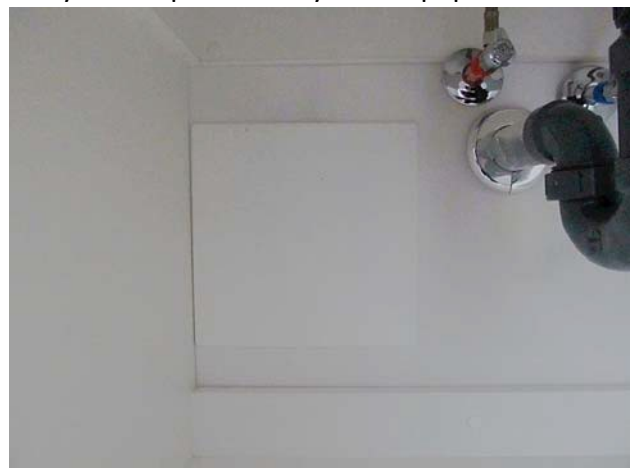
View of interior of cabinet under sink. Water shut-off valve cover plate is seen in left corner.
