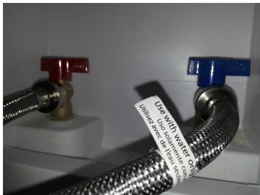
Water Shut-Off Valve
