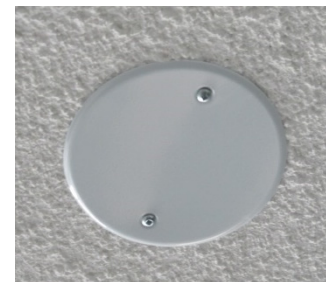
Ceiling Electrical Box
