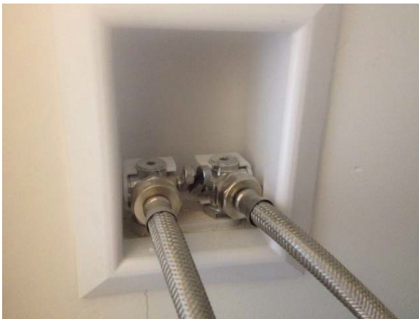
Water Shut-Off Valve
