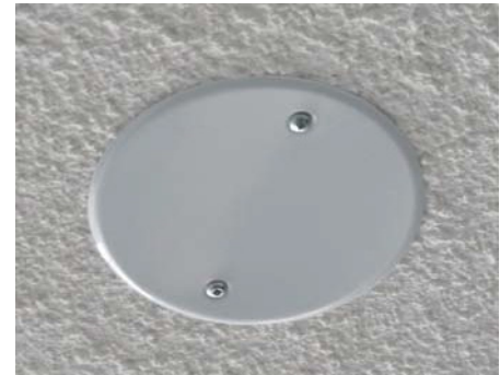
Ceiling Electrical Box
