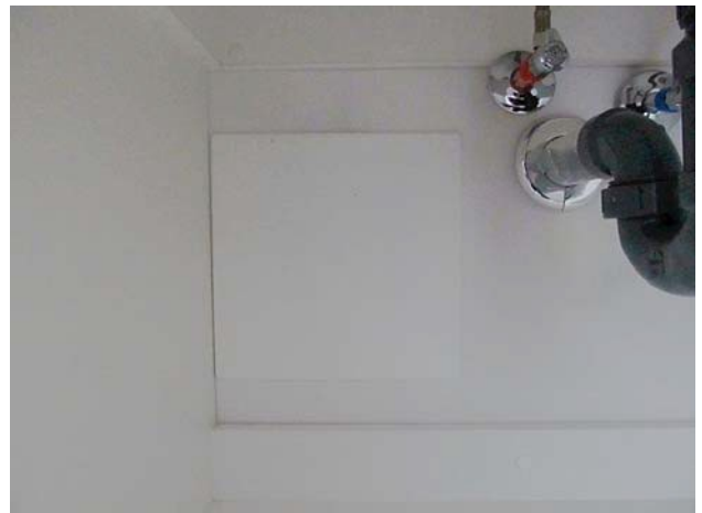
View of interior of cabinet under sink. Water shut-off valve cover plate is seen in left corner.
