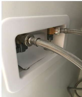
Water Shut-Off Valve
