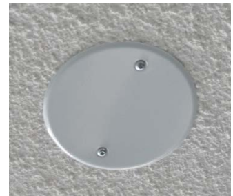
Ceiling Electrical Box
