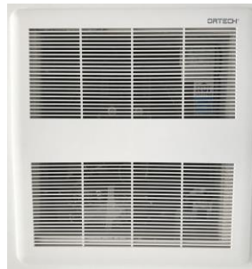
Typical bathroom / ensuite exhaust fan
